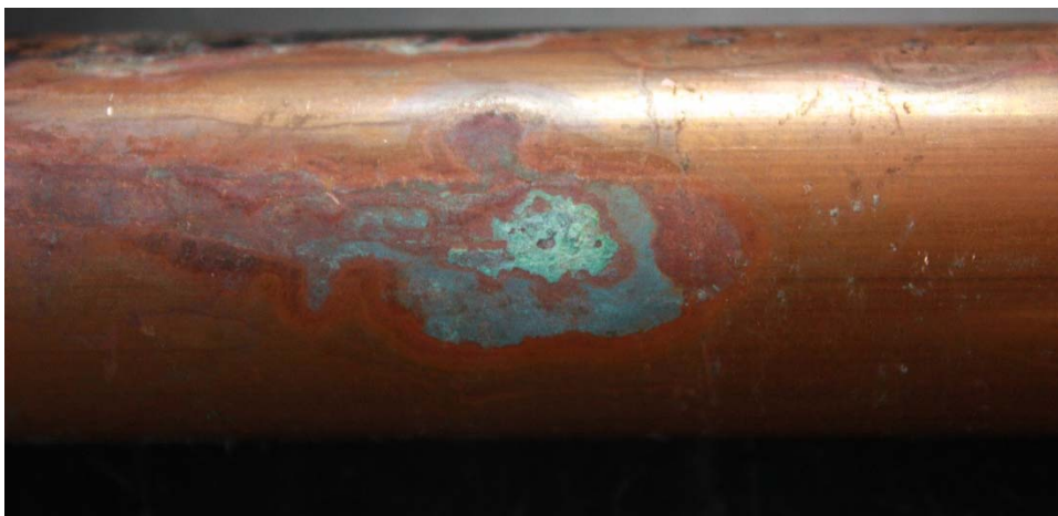
Figure A.5 – Pipe #5 interior surface (top) and exterior surface (bottom)
