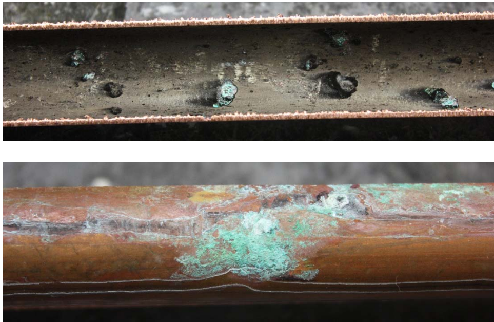
Figure A.1 – Pipe #1 interior surface (top) and exterior surface (bottom)
