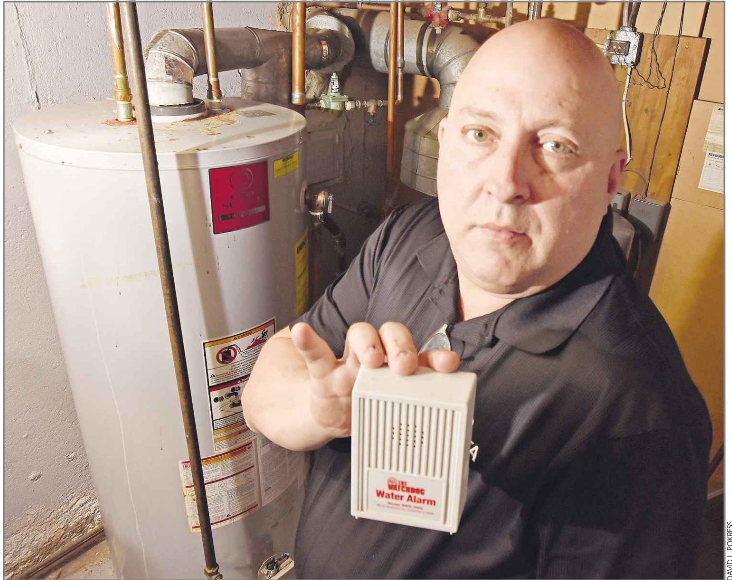
Wayne Weinstein's Plainview home has been plagued with pinhole leaks, starting with pipes attached to the hot water heater, background.
