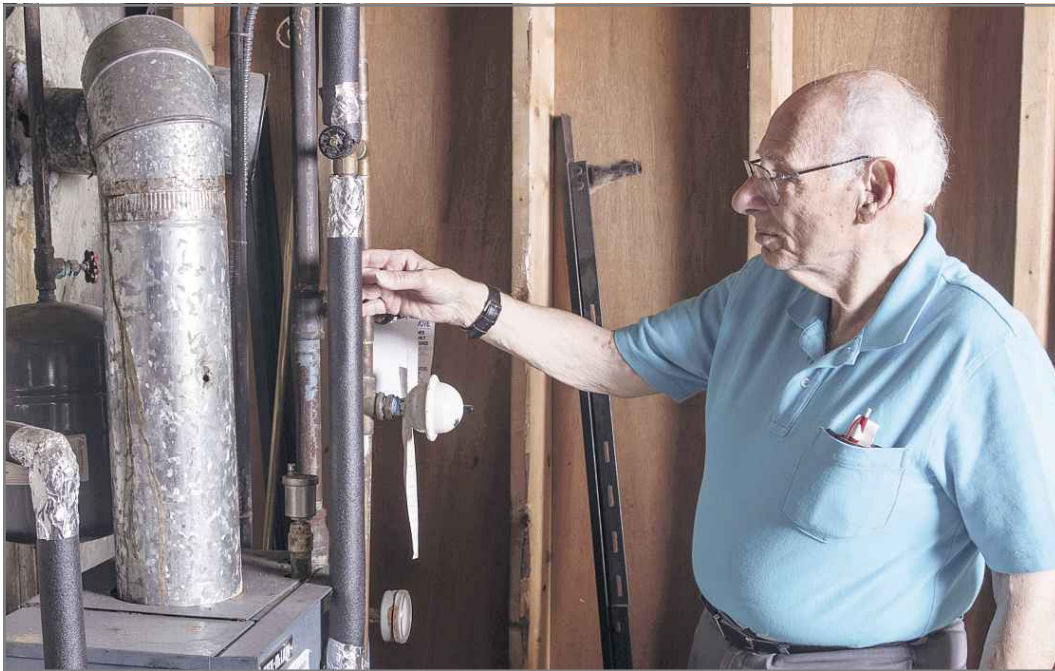
Joe Elowsky inspects the furnace inside his and wife Marsha's Plainview home last week.
