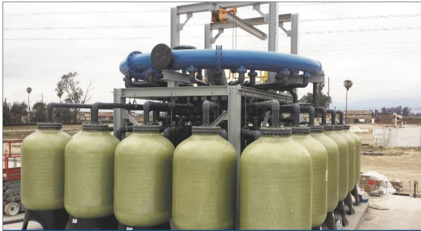
A state of the art nitrate/perchlorate system in Southern California. The Plainview Water District will be building a similar facility that will be completely contained within a new building. It will be the only treatment facility like it on the East coast.
