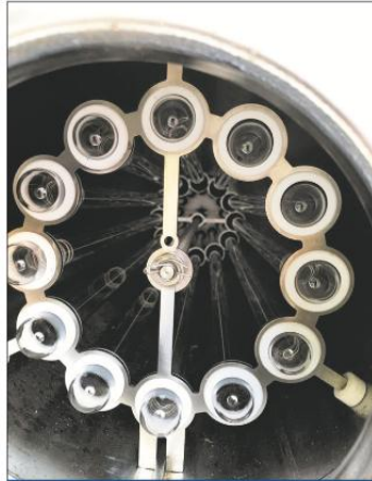
A view from inside the AOP treatment unit that uses UV light to break apart the contaminant. From there, water travels through Granulated Active Carbon units that filters out any remaining contaminant.
