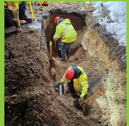
Plainview Water District crews responding to a water main break.
